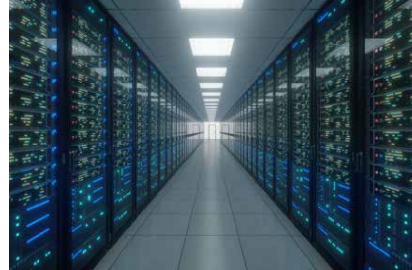
24/7 Access and Power Backup: Let nothing hinder your productivity.
